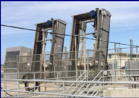
Headworks 1 Bar Screens
